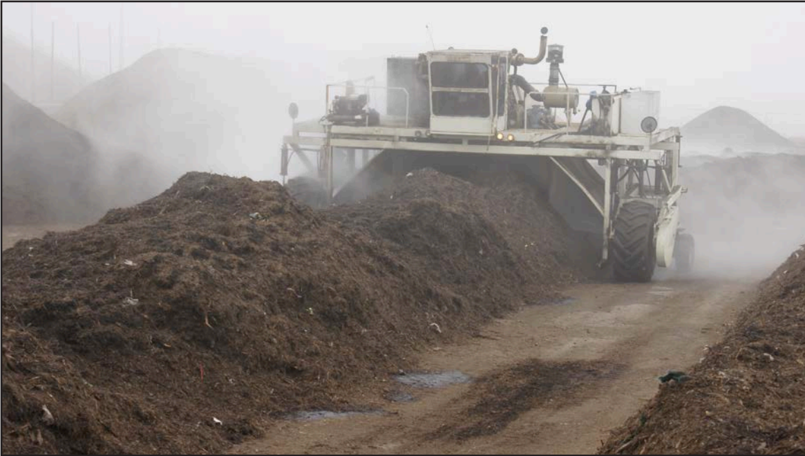
(5) Windrows are formed and are carefully monitored and kept between 50%-60% moisture content, and brought up to or above 131°F (55°C) for at least 15 days to allow involved biology to stabilize the ingredients into a living and hygienic fertility amendment.
